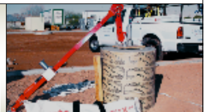
LIGHT POLE PULL
